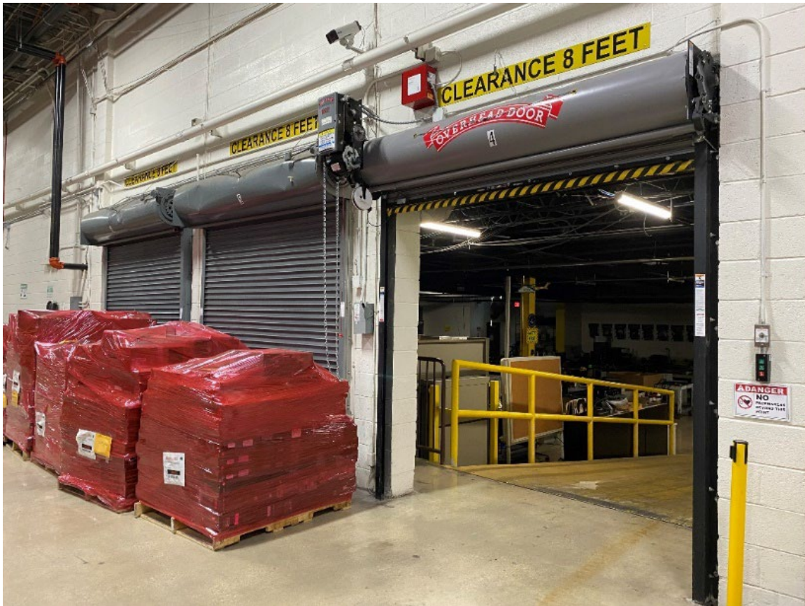
Metal Roll-Up Door to the MDT's Workspace and Non-functioning Camera
